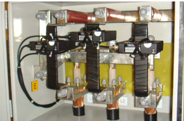
HFCT installation on SECTIONALIZED CABLE JOINTS, around ground connection cables inside link-box.
