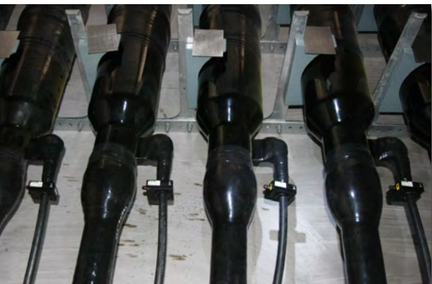
HFCT installation on SECTIONALIZED CABLE JOINTS, around ground connection cables outside link-box.
